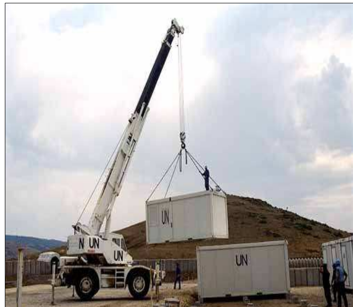
UNPREDEP Peacekeepers, part of the Indonesian Engineering platoon, use containers to construct a new observation post along the Yugoslav Border (1996). (UN Photo #187928)
